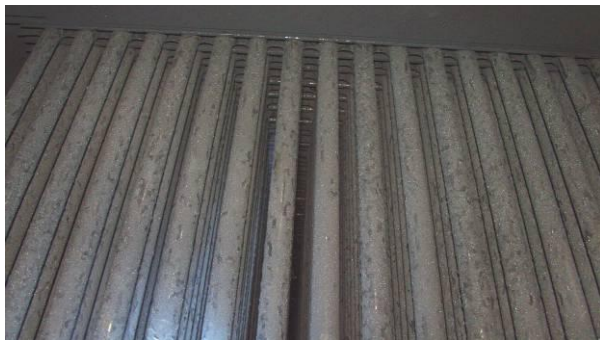
Fig. 5. HET PGV-213 power unit No 1 Rivno NNP (start-up 1980). Chemical cleaning SG provided in 2003
