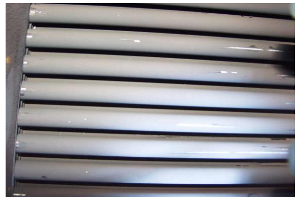
Fig. 8. HET PGV-1000M power unit No 4 Rivno NNP (start-up 2004). Chemical cleaning SG not provided
