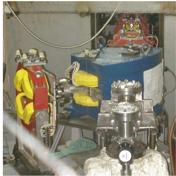
Fig.3. Installation of the injection channel quadrupoles in the project position with survey targets on the top of the elements after fodicualization at the magnetic bench
