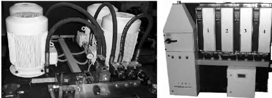
Fig. 3. 4 \times 65 LPM fixed delivery pumps (left) driven by four 30 kVA variable frequency drives (VFDs). The programmable logic controller (PLC) controlling the four VFDs ensures that only that fraction of installed 120 kVA that is really required is used at any given instant. This results in considerable reduction in energy consumed and also in energy dissipated as heat. The cooling system for this power pack is comparable to that used in conventional pumps of considerably lower capacity. Use of commercially available off-the-shelf (COTS) components such as PLCs and VFDs ensures easy maintenance with readily available spares.
