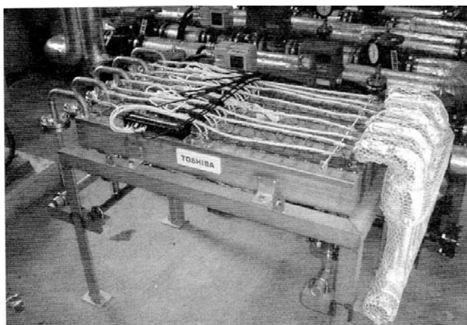
Fig. 8. Overview of 150 W class demonstration power generation system using hot springs.
