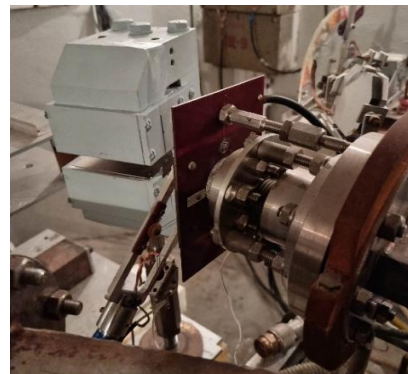
Fig. 7. The cleaning magnet was installed at the LUE-40 linac exit
