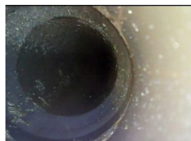
Fig. 5. The beginning of the pipe under the lower heater, the sediment layer is loose, pimples are visible
