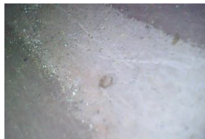
Fig. 2. Sediments on the inner surface of the pipe (lower, horizontal part), grains of calcium salts are visible
