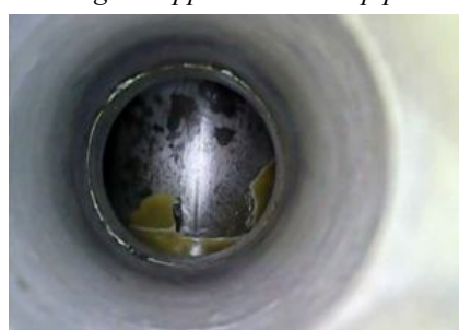
Fig. 8. The output of water from the cooler 1
