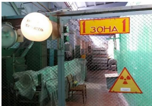
Fig. 12. Fragment of Zone 1 of the linear electron accelerator LUE-300. Detector and power supply located on the chair – point 2
