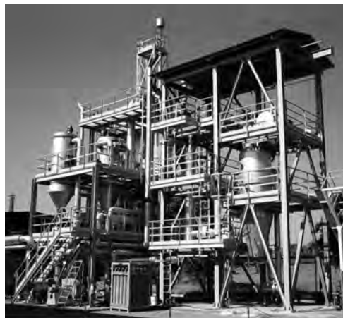
Fig.1. 500 KW th FICFB gasifier at Trisaia.
