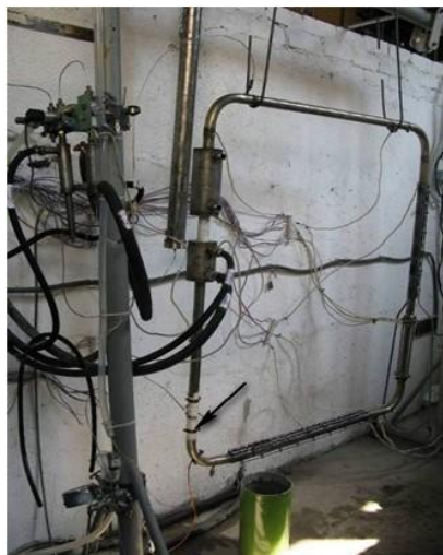
Fig. 1. Loop1a on the test bed. The arrow specifies a placement of the flow monitor
