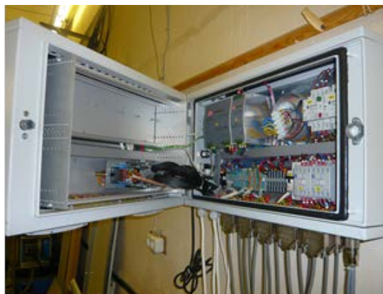
Fig. 11. The cabinet of the controller block of the automatic control system
